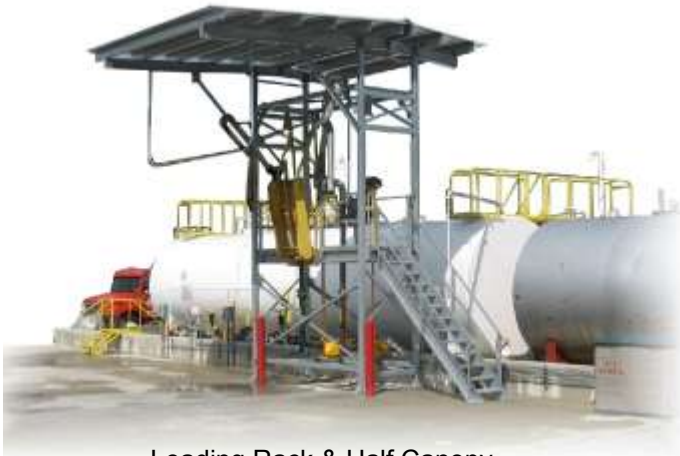
Loading Rack & Half Canopy
